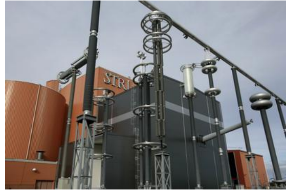
The picture shows the 800 kV HVDC long term test circuit
